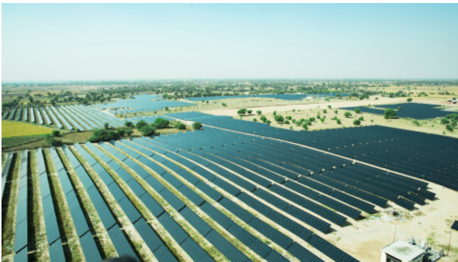
Azure Power Solar Power Plant (Photo: Business Wire)
