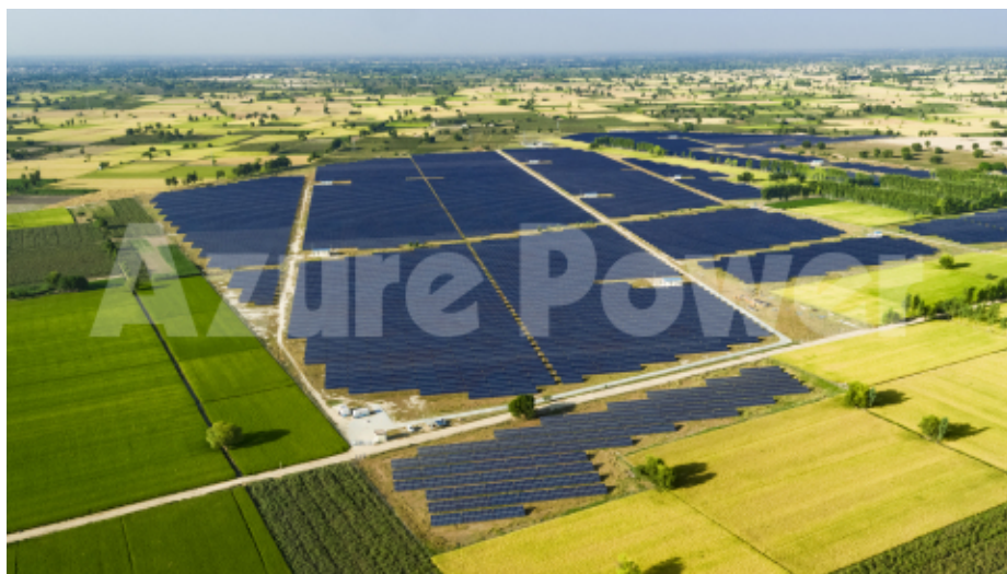
Azure Power Solar Plant (Photo: Business Wire)
