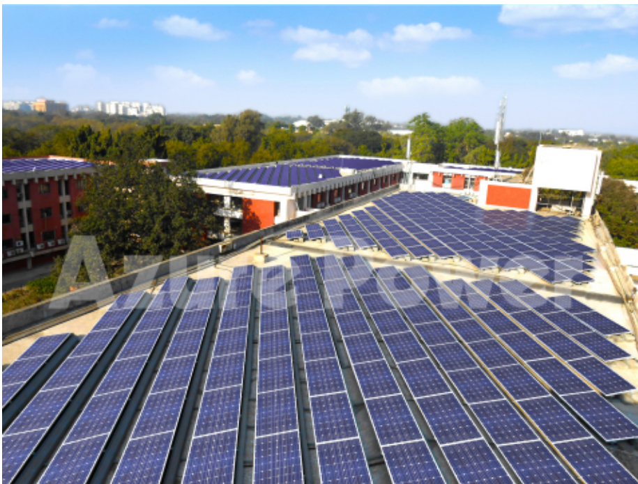
Azure Roof Power Smart City Project (Photo: Business Wire)
