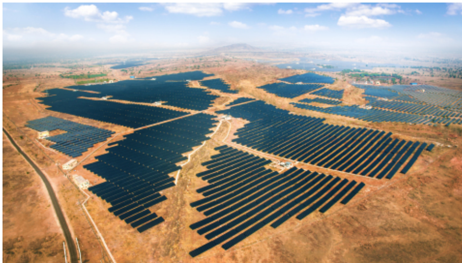
Azure Power Solar Power Plant, 100 MW, Rajasthan (Photo: Business Wire)
