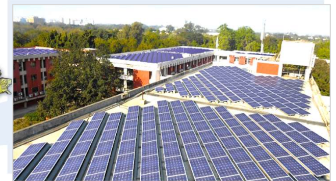
Gandhinagar | India's First MW Scale Distributed Solar Rooftop Project
