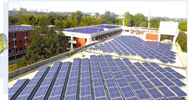
Gandhinagar | India's First MW Scale Distributed Solar Rooftop Project
